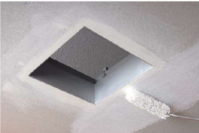
After sanding down the surface, paint over with wall colour. After suitable primer coating the fitting frame can be painted in the same wall colour.
